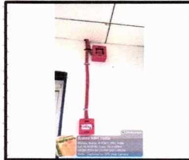
Fire Alarm System
